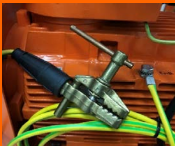
Earth Cable with Clamp.
